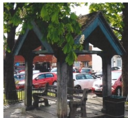
Dilapidated well prior to restoration
