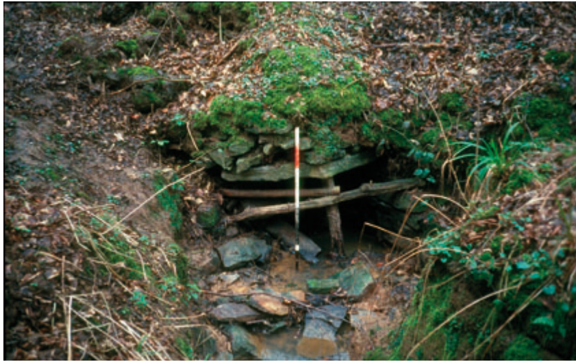
Culvert at Strawberry Wood, near Benenden in the High Weald (photo - NB)
