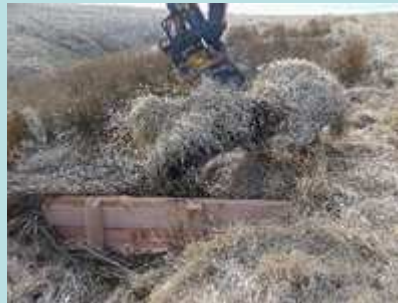
Grip blocking of drainage channels
