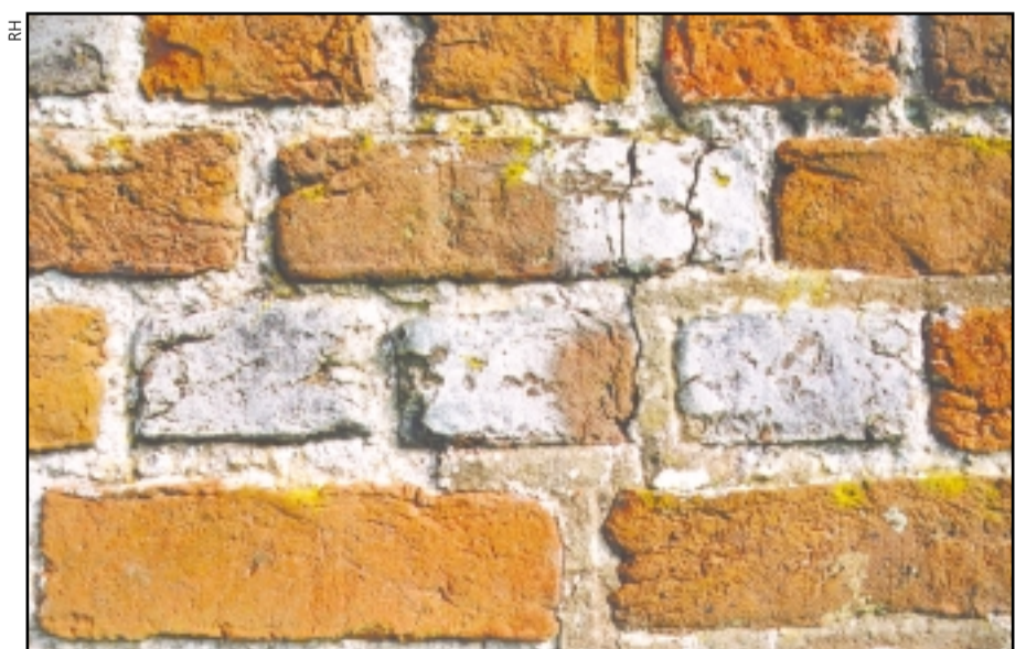
Brickwork, St John the Baptist's church, Small Hythe, Kent. Rebuilt in brick 1516-17.
